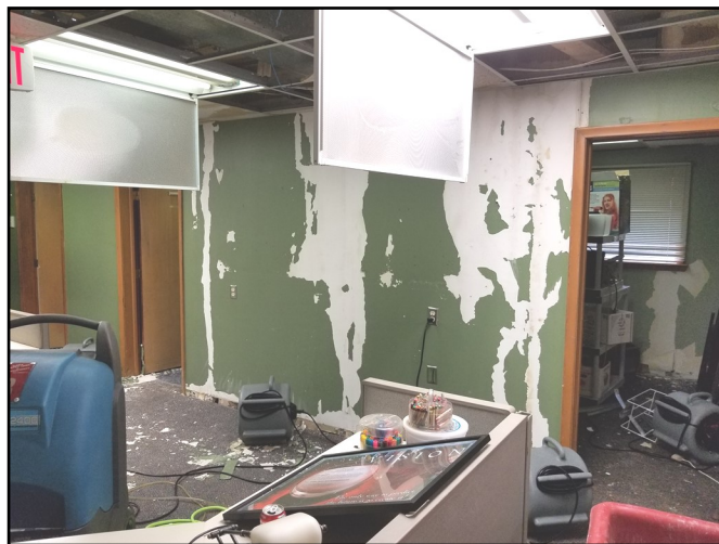
Lower Level Unit destruction from water coming through ceiling.
